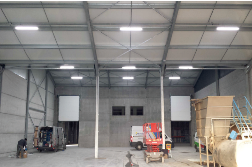
Date: April, 2016 Product: Tomline linear high bay 150W Application: Warehouse Country: Belgium
