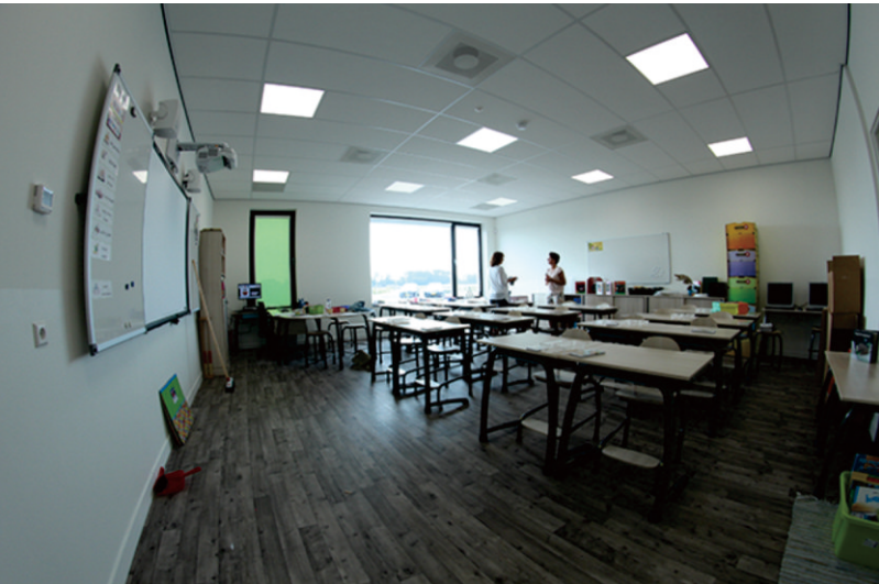
Date: April 2015 Product: LED panel light Application: School Country: Netherlands
