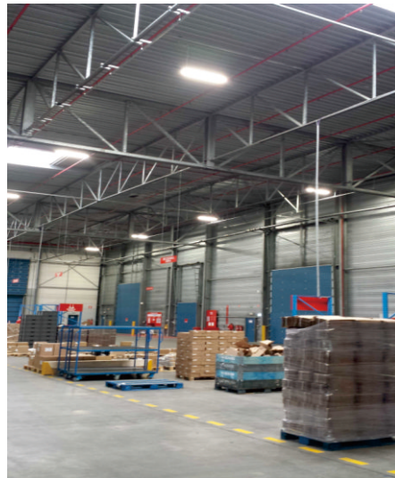
Date: March 2016 Product: Tomline linear high bay 150W Application: Warehouse Country: USA
